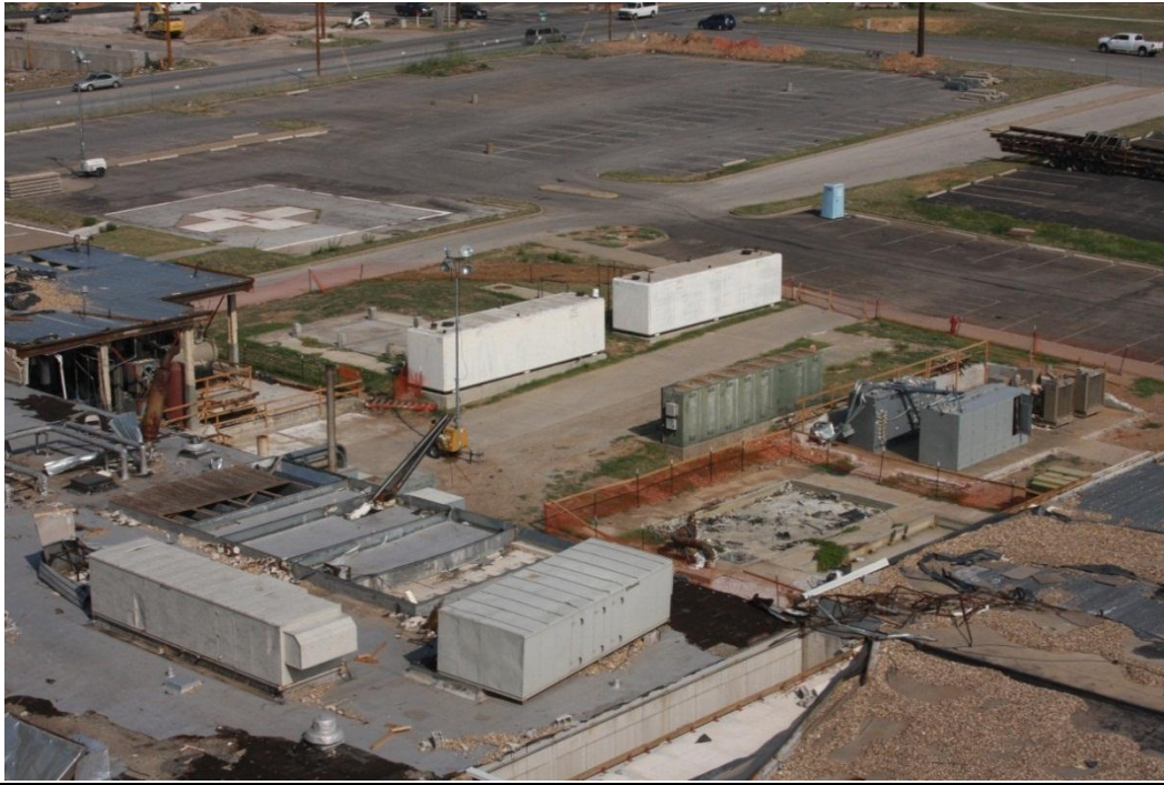
Photo 17: St. John's Medical Center – mechanical and back-up generator buildings destroyed by the tornado. Area cleaned prior to site visit.
