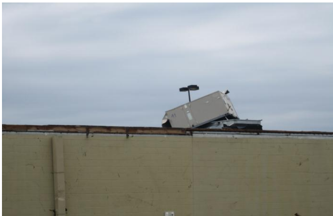
Photo 34: Architectural elements and mechanical units dislodged during high winds.
