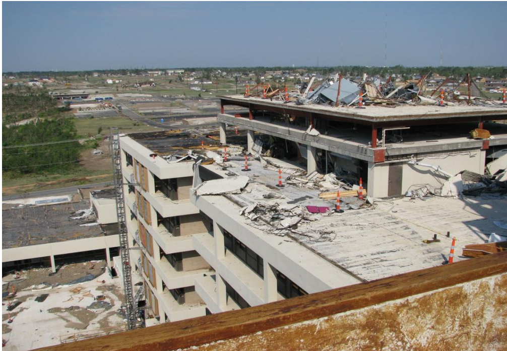
Photo 16: St. John's Medical Center, penthouse at concrete frame building with mechanical penthouse constructed of structural steel and light weight concrete on metal roof deck.
