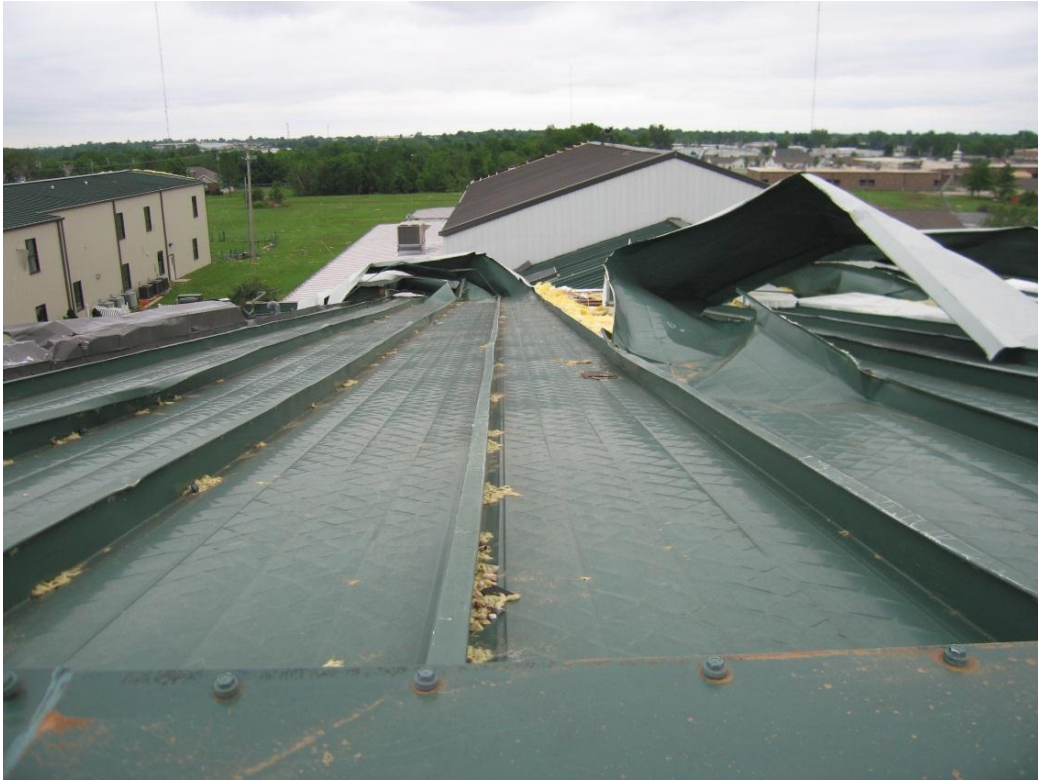
Photo 9: Roof Damage to north slope of sanctuary.
