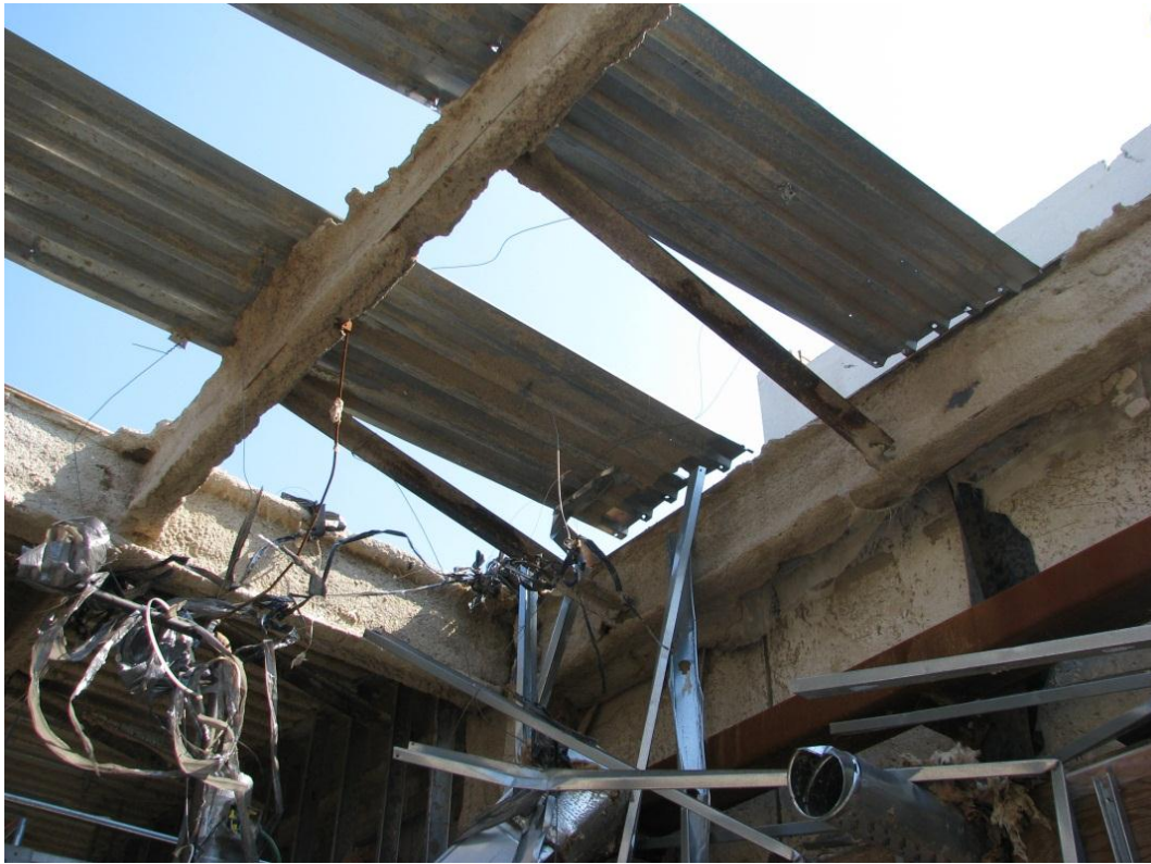
Photo 23: St. John's Medical Center –Failed metal roof deck to structure connection.
