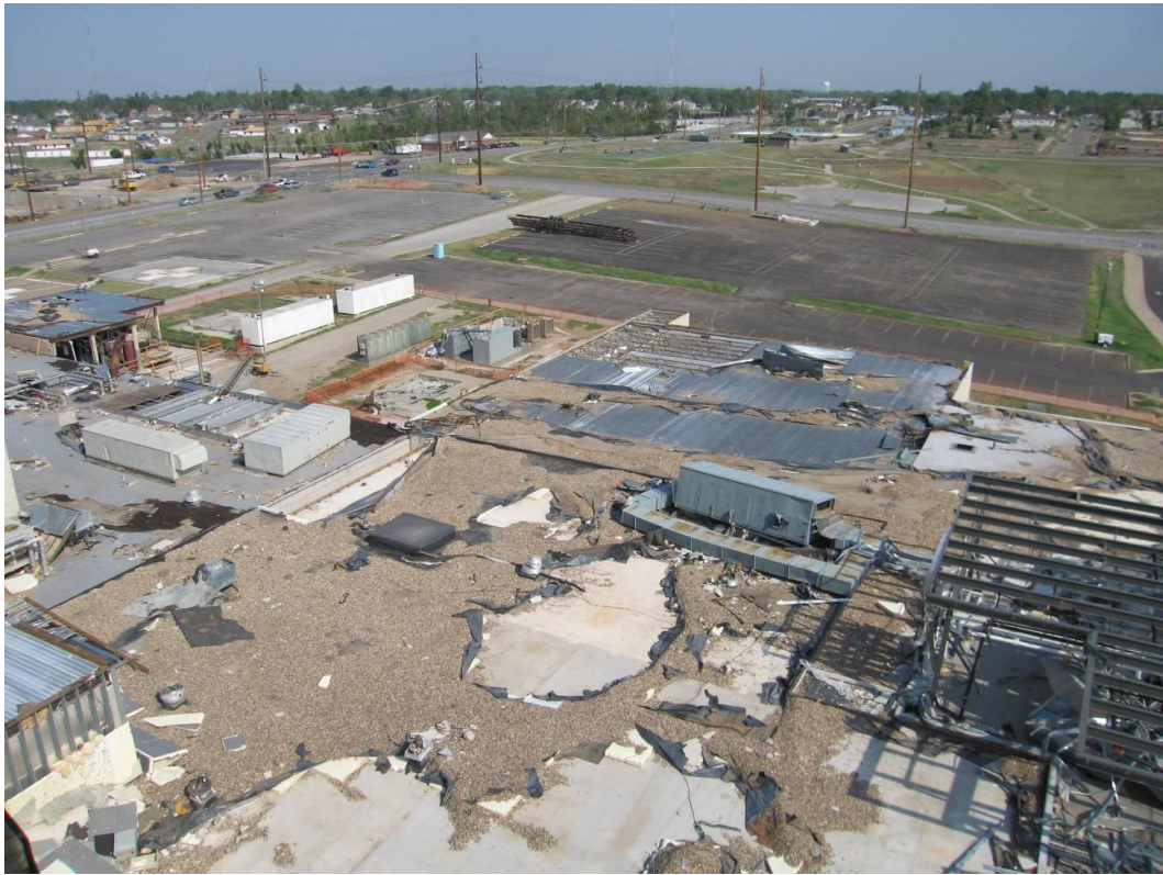
Photo 15: St. John's Medical Center, damage to penthouses and roof equipment. Note the missing metal roof deck on penthouse, looking NW.
