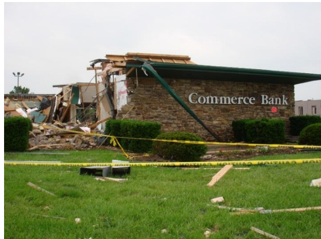
Photo 4: A non-residential wood frame structure near the center of the tornado.
