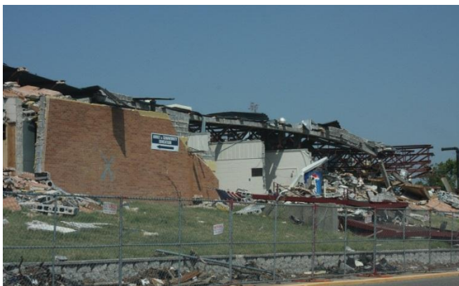
Photo 36: Hard wall collapse to the outside of building, with second level roof collapse.
