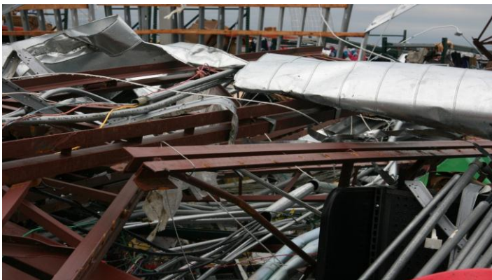
Photo 30: Arc spot welds on top of steel joist where metal deck pulled free. Failed weld at joist bearing with distorted clip angle. Joist remained inside the building footprint.
