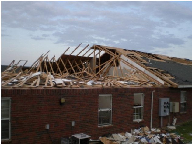
Photo 1: Note the anchorage of the trusses to the sidewalls in this building: the top chord of the truss broke before the anchorage failed.
