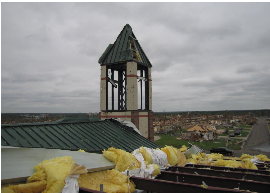
Photo 12: The free standing church steeple exhibiting the loss of cladding, while the main structure system remains intact.
