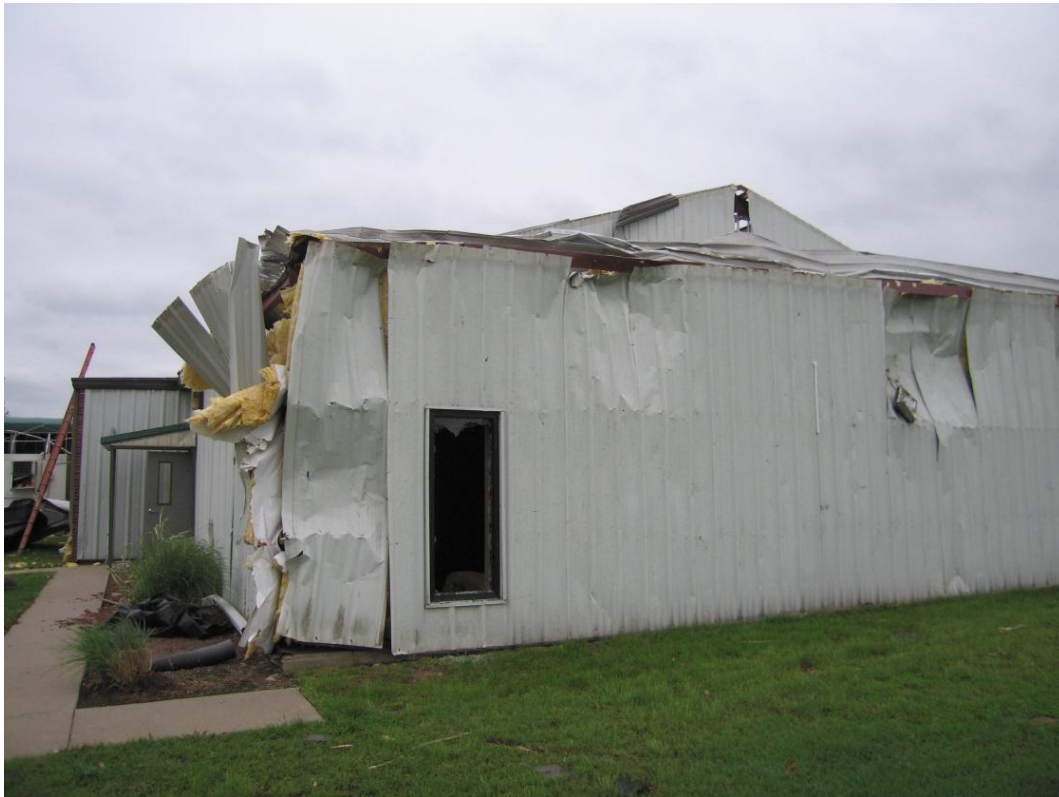
Photo 11: Damage to northeast corner of building.
