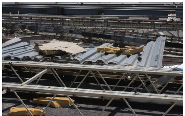
Photo 37: 18 gage metal deck attached to joist, after demolition of building struck by the tornado.
