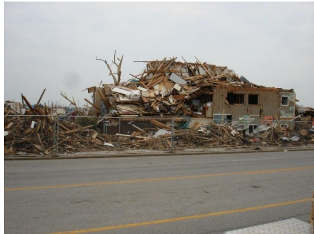
Photo 2: Destruction of the main roof system, second story, but the redundancy of the wood structure prevents total collapse.
