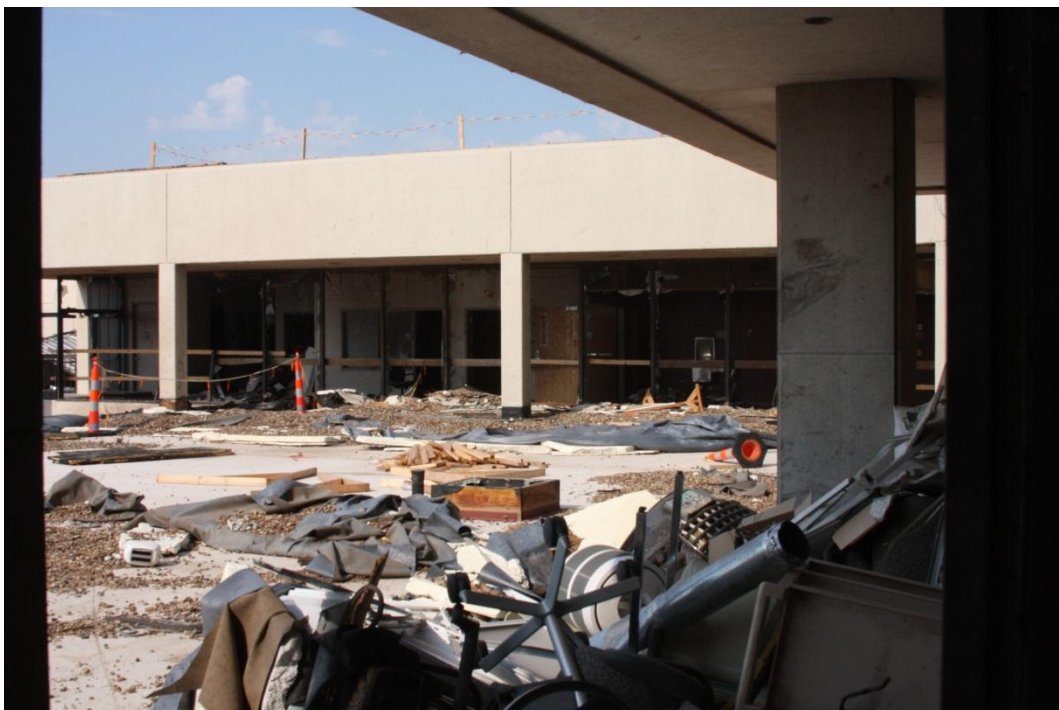
Photo 14: St. John's Medical Hospital damage, note the ballasted roof, light weight concrete on roof and curtain wall glazing system destruction.
