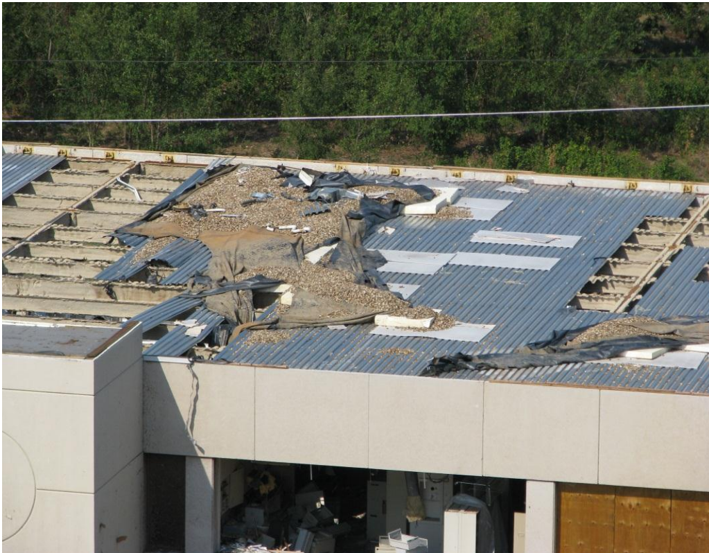
Photo 22: St. John's Medical Center MOB - Steel Frame Building with missing and damaged ballasted metal roof decking.
