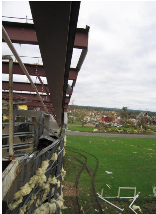
Photo 8: Cold Formed Metal Stud Failure due to poor attachment to the underside of the purlin overhang.
