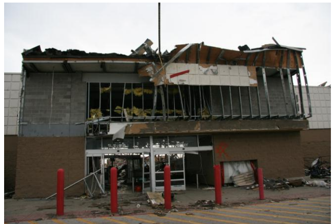
Photo 35: Architectural elements and cold formed steel stud framing damage.
