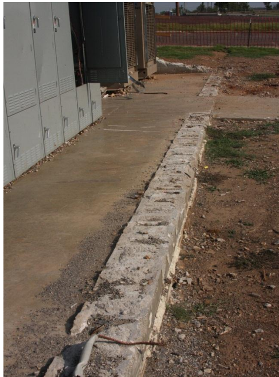
Photo 18: St. John's Medical Center – The mechanical and back-up generator masonry wall buildings appear to lack sufficient reinforcing bars. Note: the area had been cleaned up prior to our investigation.
