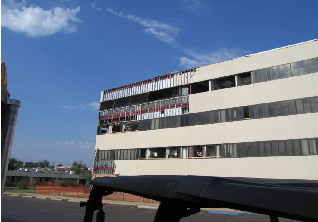
Photo 19: St. John's Medical Center - Steel Frame Building - damaged glazing and exterior cladding
