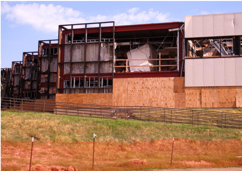
Photo 20: St. John's Medical Center – Steel Frame MOB - damaged glazing and cladding
