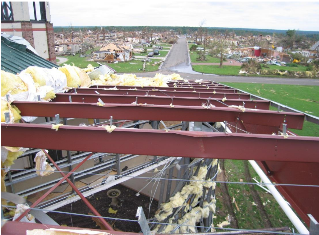
Photo 10: Purlin damage at the east end of the sanctuary building, along with failure of the exterior wall framing.
