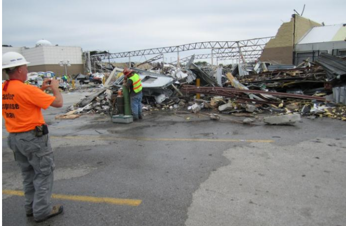
Photo 32: Upward bow of joist girder due to overstress loading of uplift pressures during tornado.
