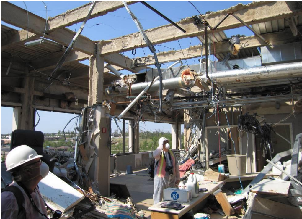
Photo 21: St. John's Medical Center MOB - Steel Frame Building with missing and damaged ballasted metal roof decking.
