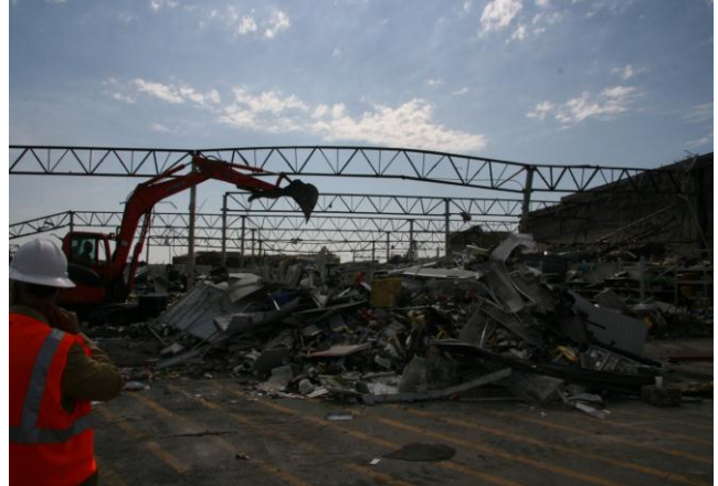
Photo 33: Upward bow of joist girder due to overstress loading of uplift pressures during tornado.
