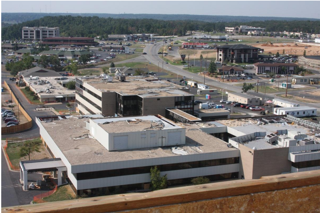
Photo 24: St. John's Medical Center MOB - Steel Frame Buildings with missing and damaged ballasted metal roof decking.
